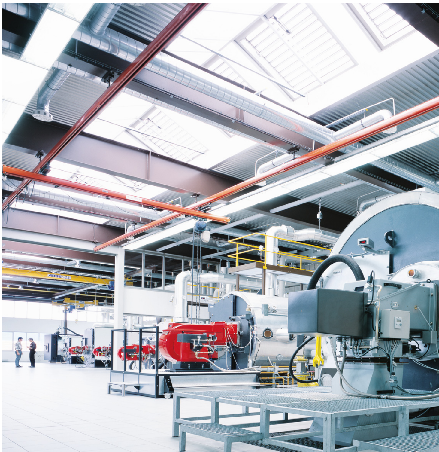
Test beds in the Weishaupt Research and Development Centre
